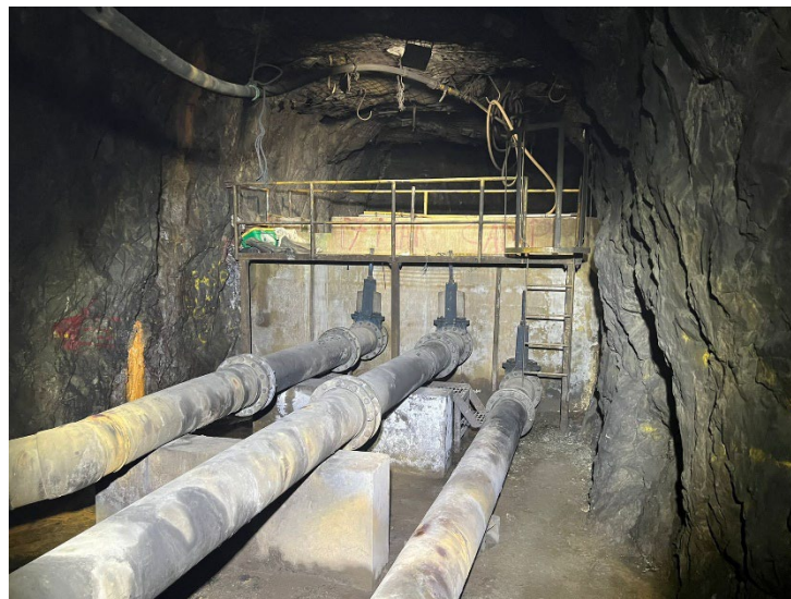
Figure 24.3.39 Central Dewatering System 1185 m RL
