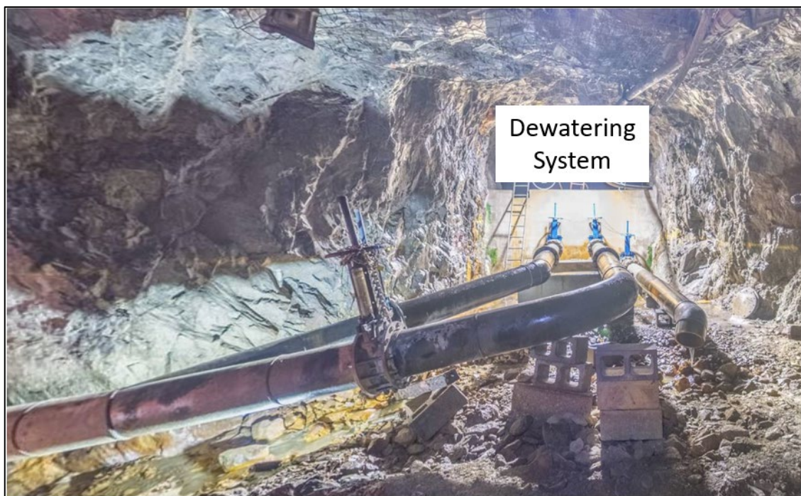
Figure 16.10.3 Central Dewatering System 1185 mRL
