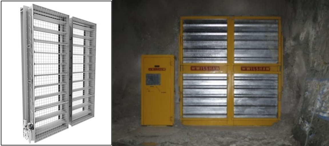
Figure 16-46 Example of Ventilation Louvres care of Clemcorp and Wilshaw
